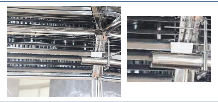
Temperature and Humidity Sensor
